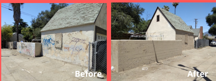
Graffiti Cleanup on West 9th Street (Ward 1)
