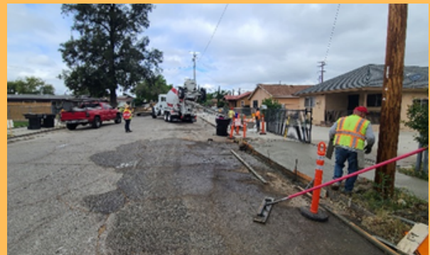
Crews working on King Street as part of Citywide repaving project (Ward 1)
